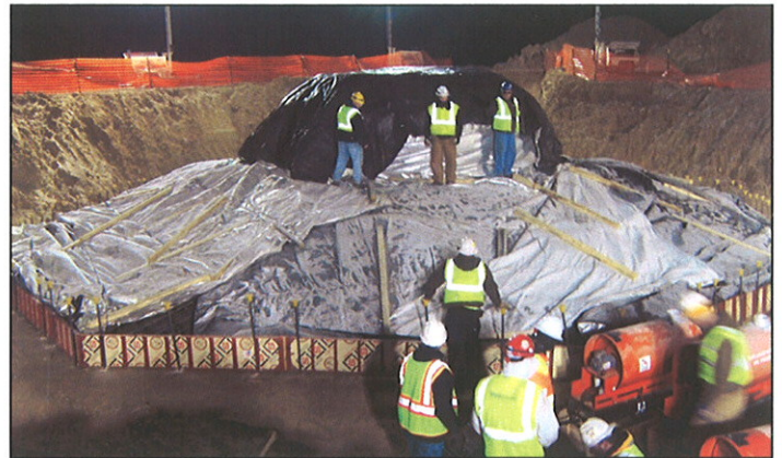
Building & Earth Sciences tests the materials used to support the massive wind turbines.
